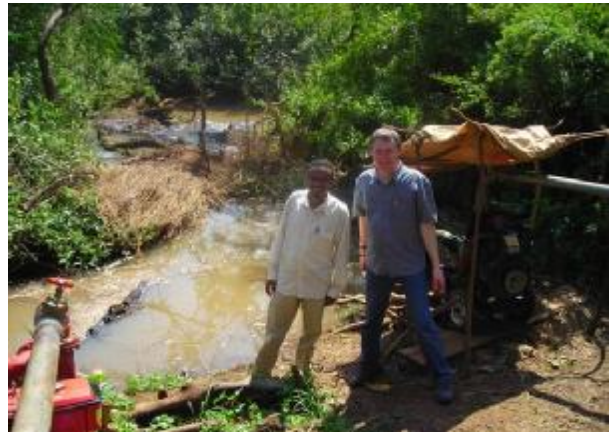
Irrigation system used by the Agricultural Research Centre to grow off-season crops.
