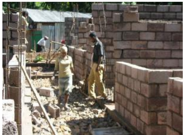
An earlier phase in the building programme for the Eye Clinic back in December.
