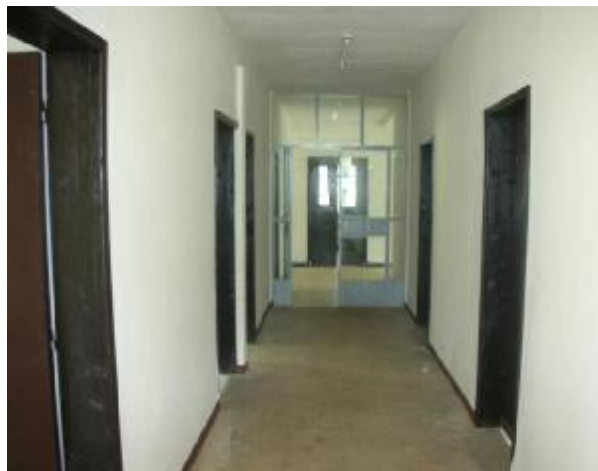
The interior is now ready. Equipment and staff are on their way—and soon, patients.
