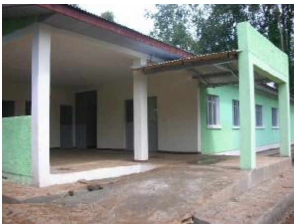
The main entrance to the new Eye Clinic in Nekemte. Doors to open very soon!
